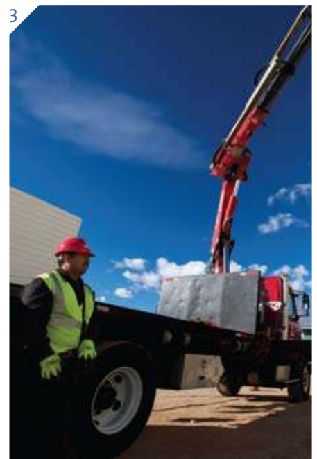
3. Distribution: Ricardo Alvaros of Allied Building Products unloads insulation at a new school construction site in Boulder, Colorado, USA.
