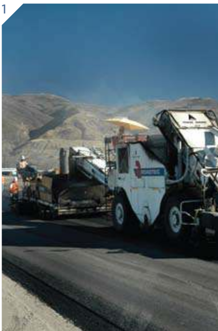
1. Materials: Staker Parson supplied four million tonnes of product in addition to completing all of the asphalt paving for the Legacy Parkway upgrade in Davis County, Utah, USA.
