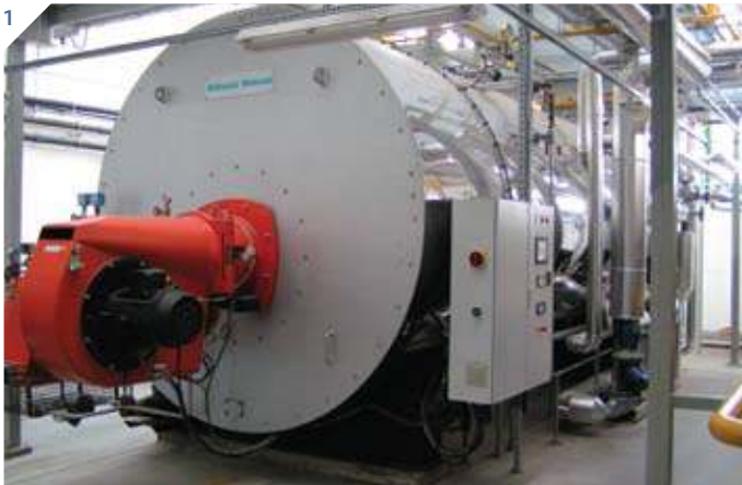
1. A new gas-fired boiler, which contributes to reduced energy use, has been installed at Prefabet's Reda aerated concrete production plant in northern Poland.
